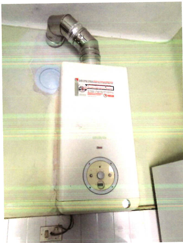
11 – caldaia a gas
